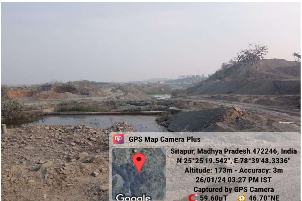
Dumping of dust and bridge constructed at Babedi Naala, Sitapur, causing disruption of natural flow of Naala. Photo dt. 26/01/2024
